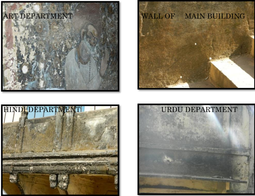
Fig.1.Different deteriorating site of KRG College
